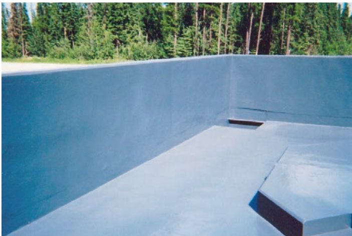
Stonchem 403 met all performance and durability expectations for Alberta Pacific's secondary containment areas.
